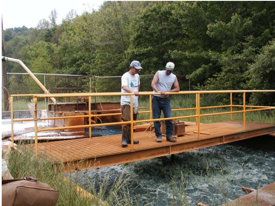
Photo 15: Part of an active AMD treatment plant on Kanesh Creek, run by International Coal Group . Hydrated lime is mixed with AMD just before it enters the mixing chamber. A large propeller under the metal walkway mixes air into the AMD to oxidize iron. After mixing, AMD flows into several large settling ponds.
