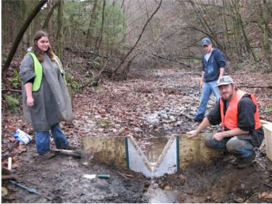
Photo 20: Rebecca Rhodes, Ben Brinkman and Martin Christ show off the newly built and installed weir placed in an unnamed tributary to Sandy Run in the Kanawha Creek sub-watershed.
