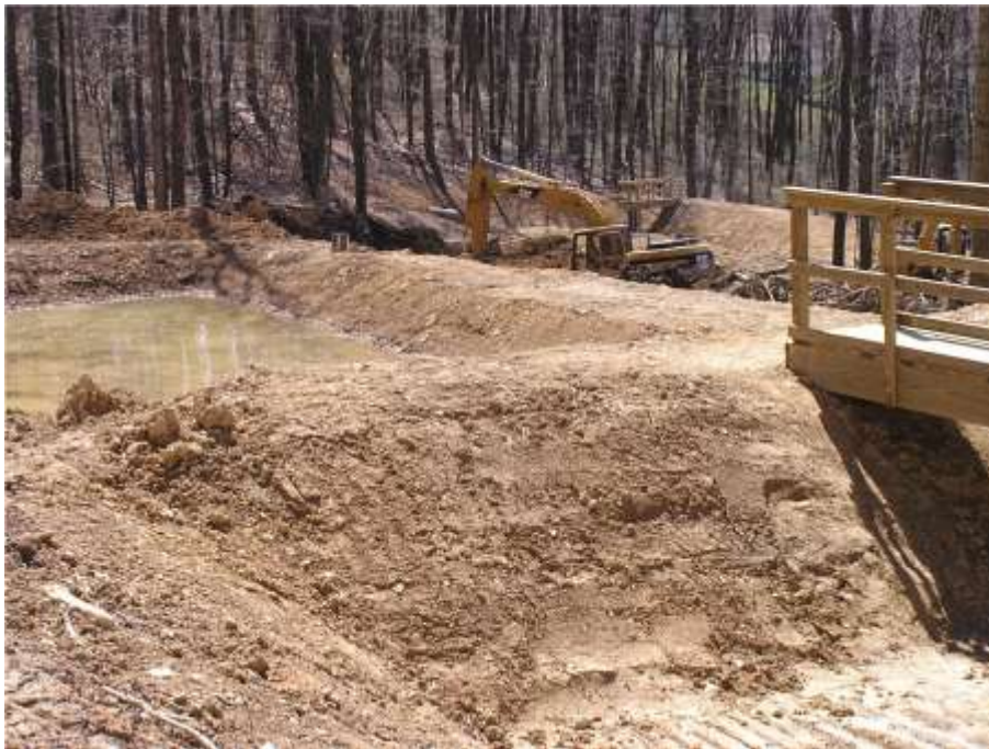
Photo 21: Construction of an AMD remediation project at VP12 in the upper portion of the Deckers Creek watershed.
